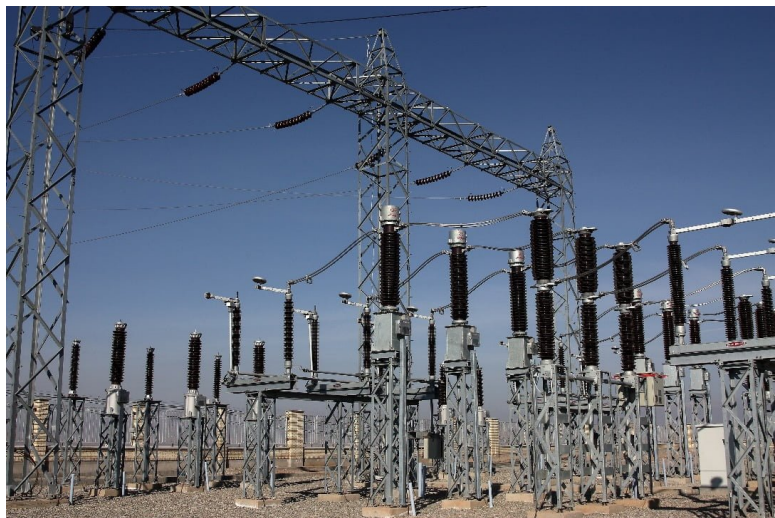
Power Supply to Karamabad Poldasht Pumping
